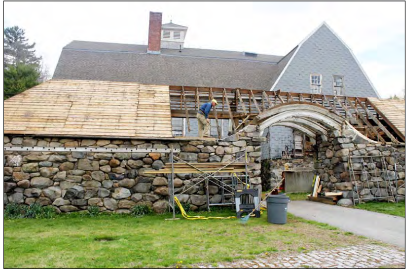
Broderick Stable renovations are expected to be completed by the end of June.
