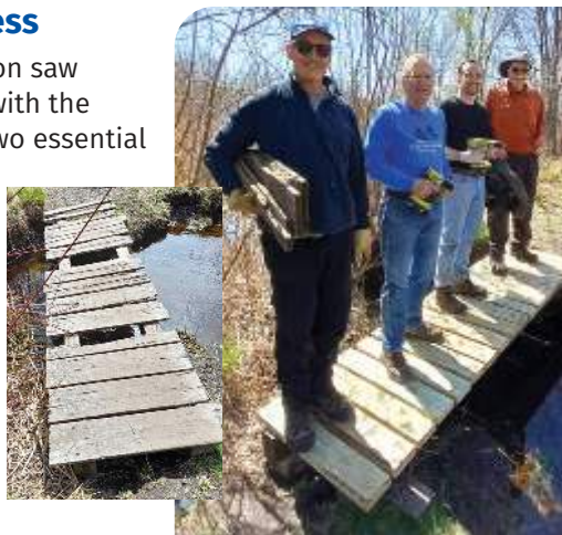
The bridge at Fowl Meadow (left) before our volunteers got to work on it.
